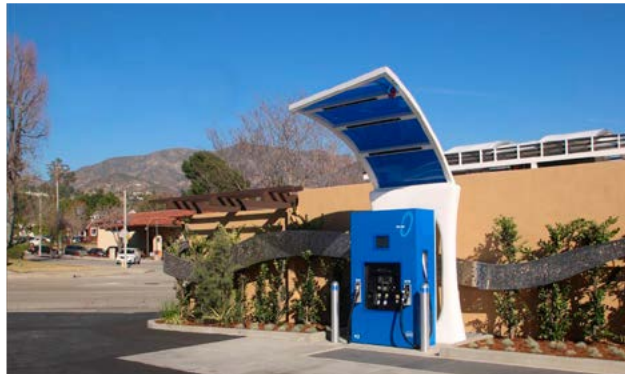
Public hydrogen fueling station in California, U.S.
