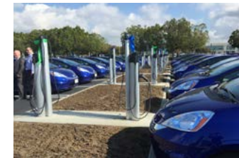
EV Charging Stations at American Honda Motor Co. Inc.
